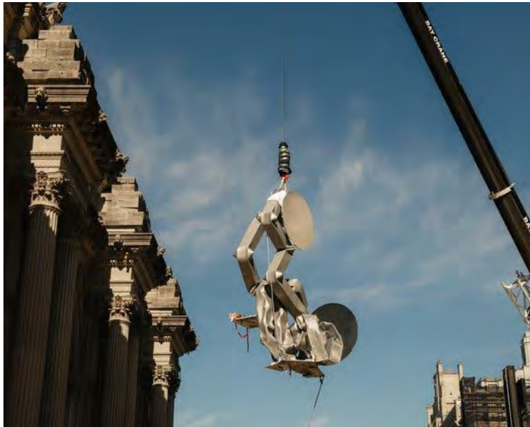
Being hoisted into position on the Met's facade during the installation process. The works have an unexpected lightness that belies the steel, and the crunch and crush of their making. Credit... George Etheredge for The New York Times
